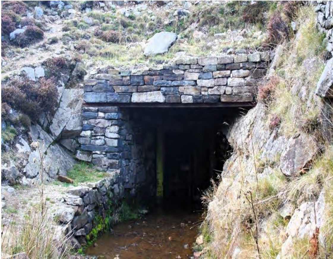
This shows the re-opened entrance in August 2011 virtually as it was at closure,. We even replaced the rail in the roof exactly as it was at closure, with English Heritage providing £3000 for the materials
